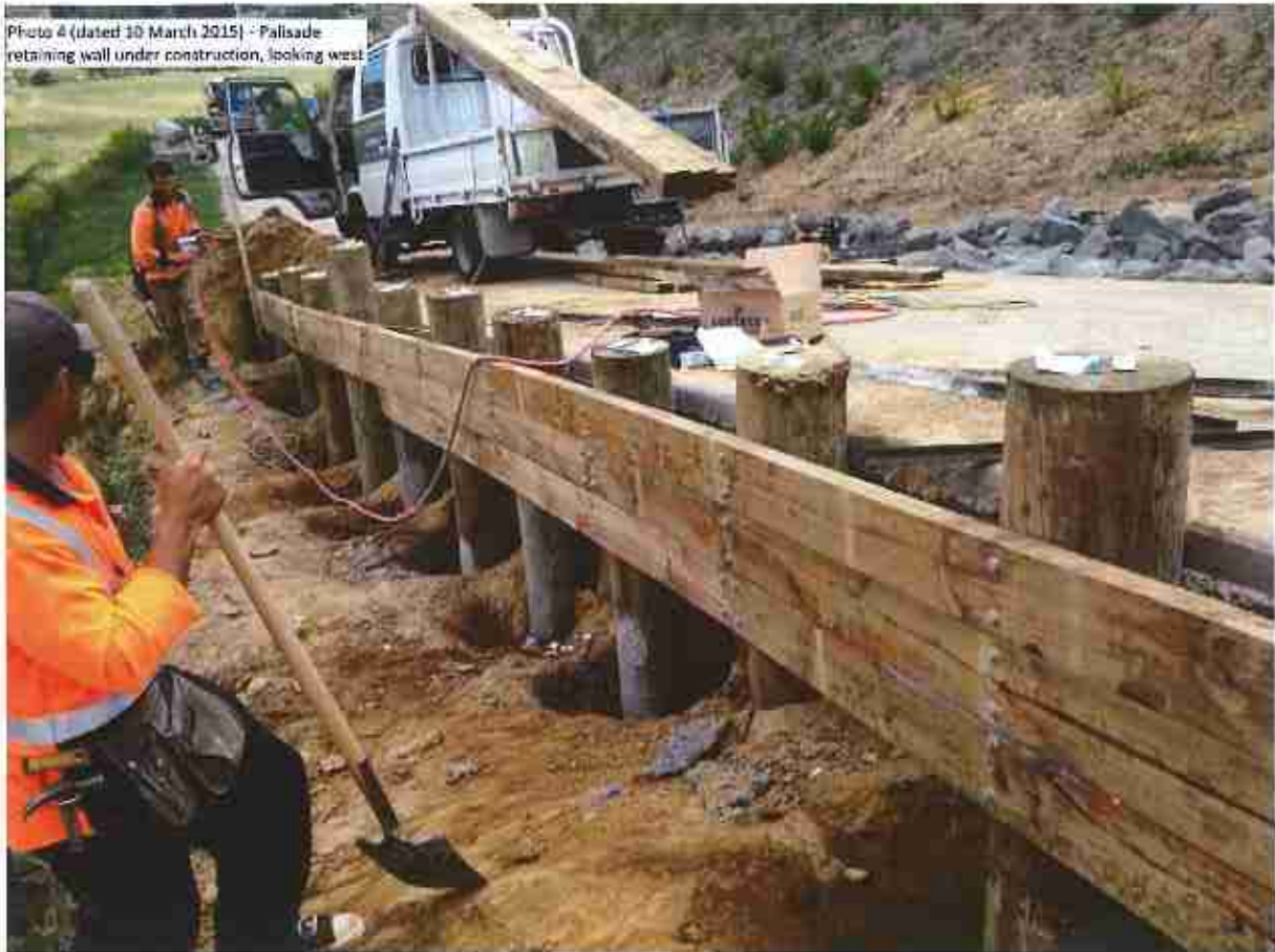
Photo 5 (dated 10 March 2015) - Timber posts at 1.0m centre to centre spacing
